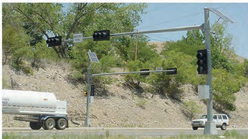
Three 3-section signal heads (solar powered). Lights are green until fire station activates.
