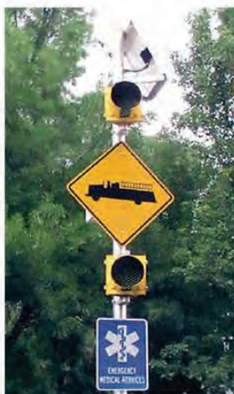
Typical solar powered EVCS.
